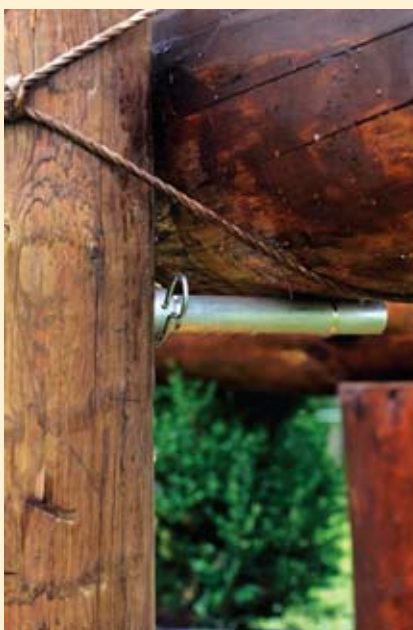
BELOW: This pin was not installed correctly.
